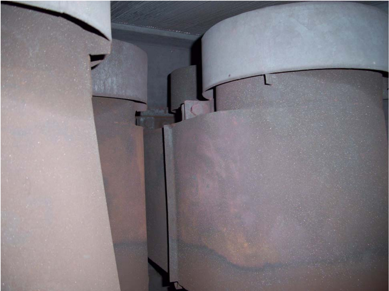
Photo 5: The whitish sparkling particles seen above the normal water level in the drum. This must be due to foaming created by excess phosphate chemical dosing in the drum. The dosing had been on when the boiler was under slumped condition.
