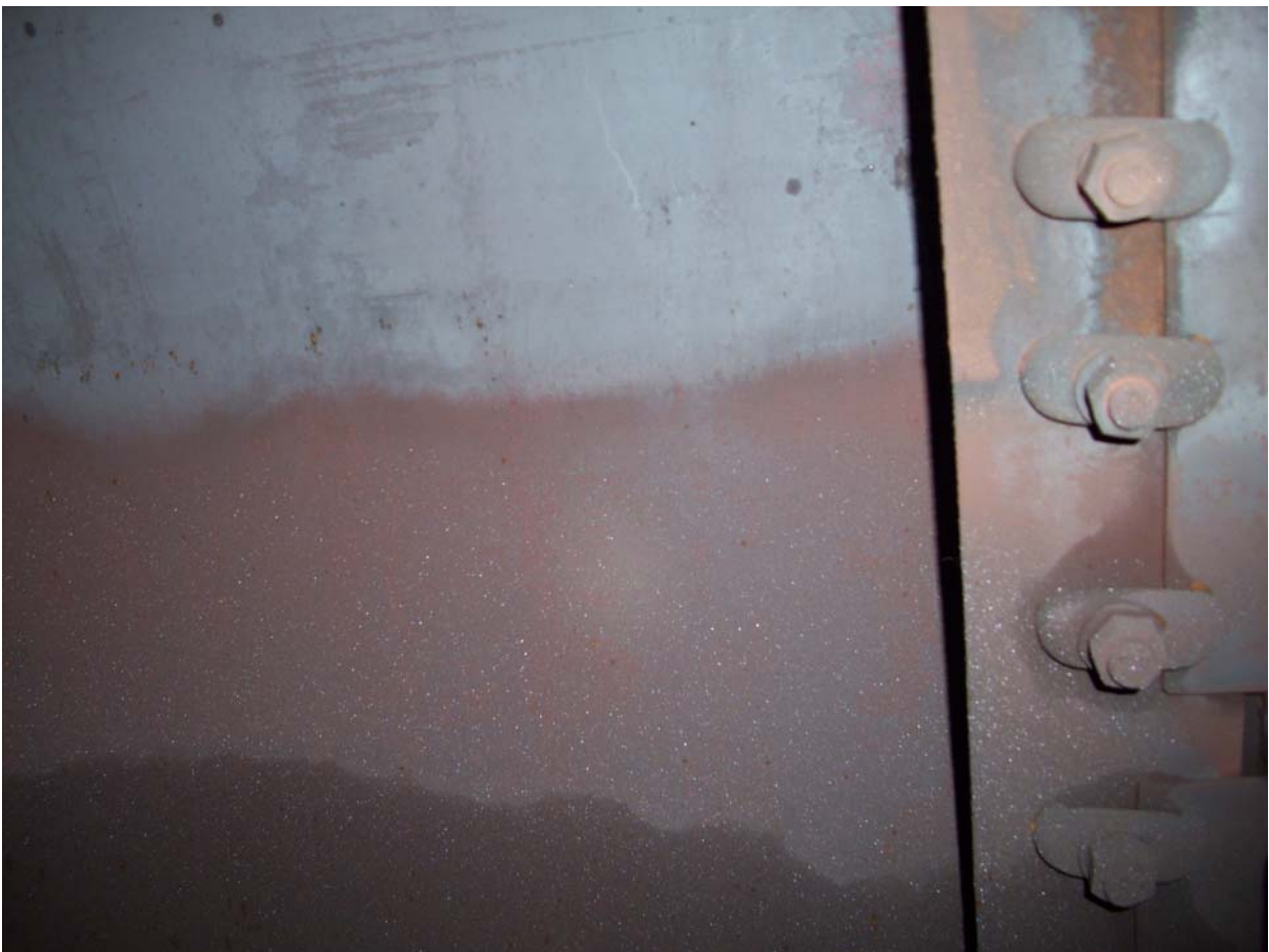
Photo 7: The boiler water chemistry had not been alright. The boiler water regime had been outside the even the coordinated phosphate control curve.
