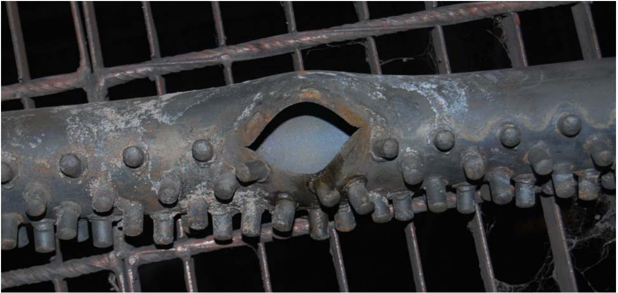
Photo 1: This is the bed SH tube failure experienced. The failed portion is in the 3 rd compartment. The edge of the failed portion of the tube is thin in nature. This indicates there has been sudden overheating situation.
