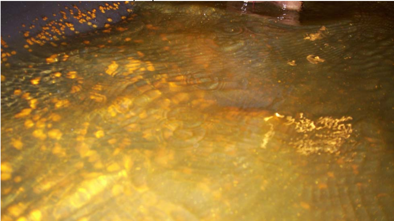
Photo 10: Presence of mud in the boiler water. The back filling of SH to be practiced to avoid carryover of dirt to SH sections.
