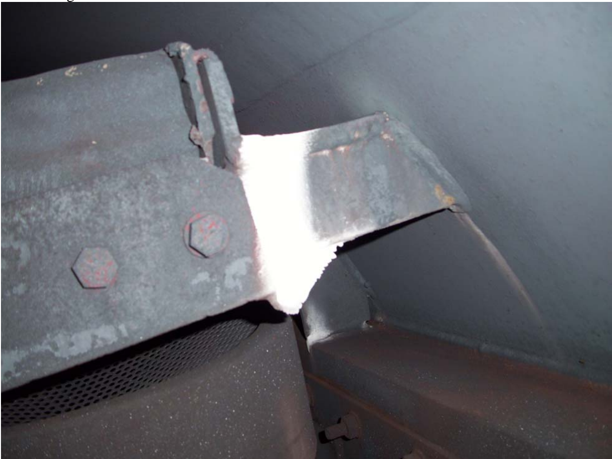
Photo 2: The drum is with the mark of excess of phosphate in the drier area.
