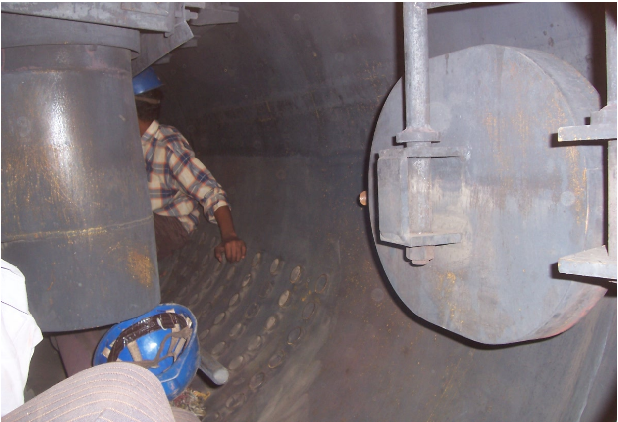
Photo 11: This is a boiler wherein the drum internal surface & turbo separators indicate the perfect boiler water chemistry.
